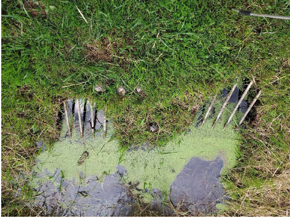
Figure 4: Tract C Outlet with standing water
