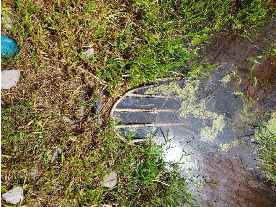
Figure 1: Tract D outlet filled with standing water
